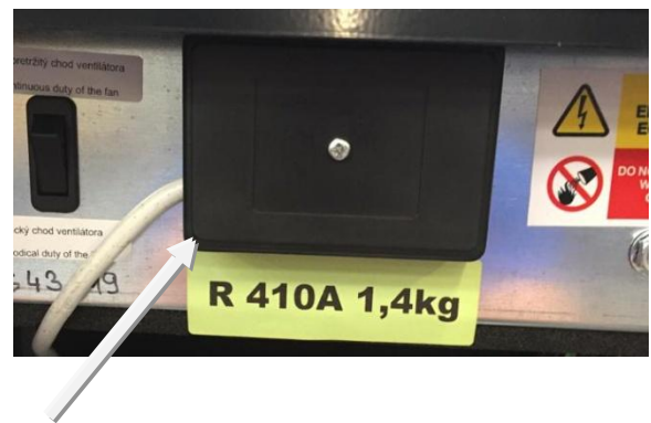
The mains terminal block is located in this black box
